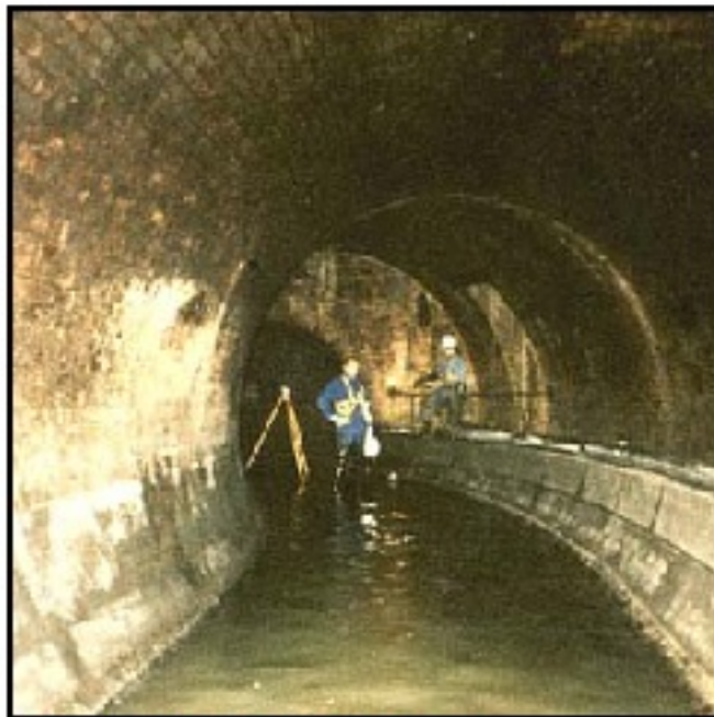
Storm relief sewer
